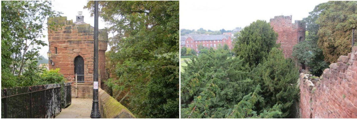
Bonewaldesthorpe's Tower and the Water Tower right, including the damaged spur wall.
